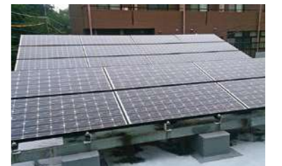
Solar panels installed on store rooftops.
